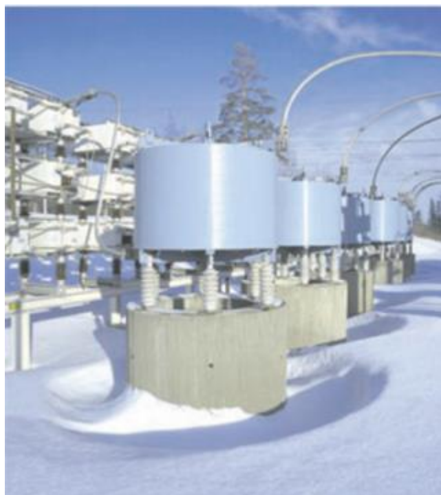
AC filter reactor
