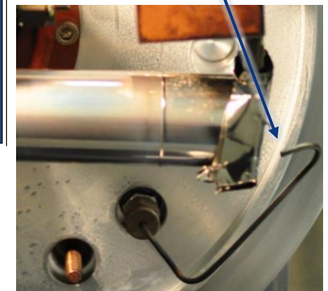
Gas line rupture
