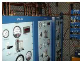
Gas delivery to 6 locations
