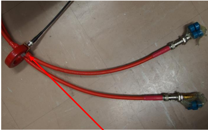
A single current transformer to measure 2 pulses, with opposite polarities.
