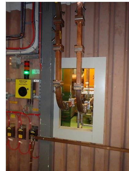
Waveguides from building 2001 to 2010
