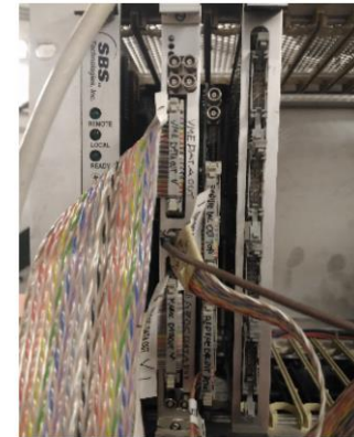
Figure 5: New VME board compact communication board, cabled to the tagging modules via flat cables, and the VME side of the SBS (Bit3) controller, installed in the BTF experimental area.
