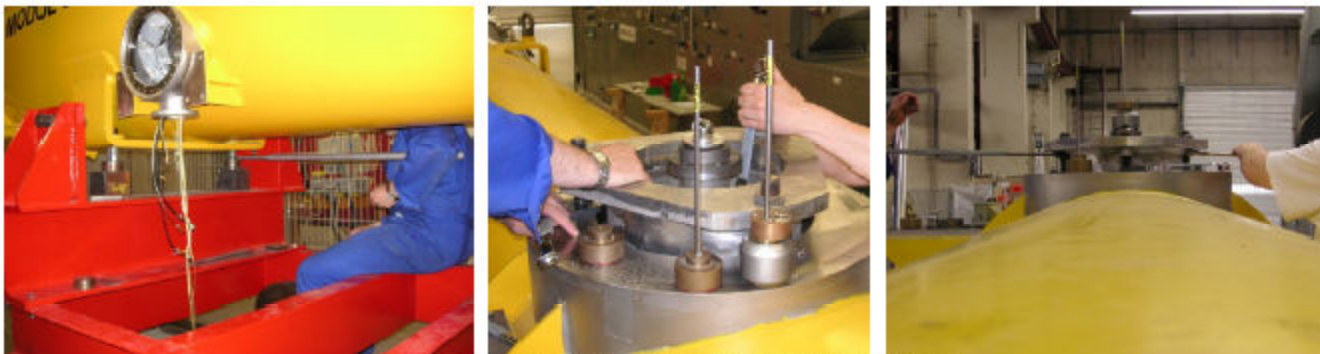
Figure 71: Adjustment of height and rotation (left: vessel rotation and height, middle: position of cold mass, right: rotation of string; middle and right action are done while measuring with Laser tracker)
