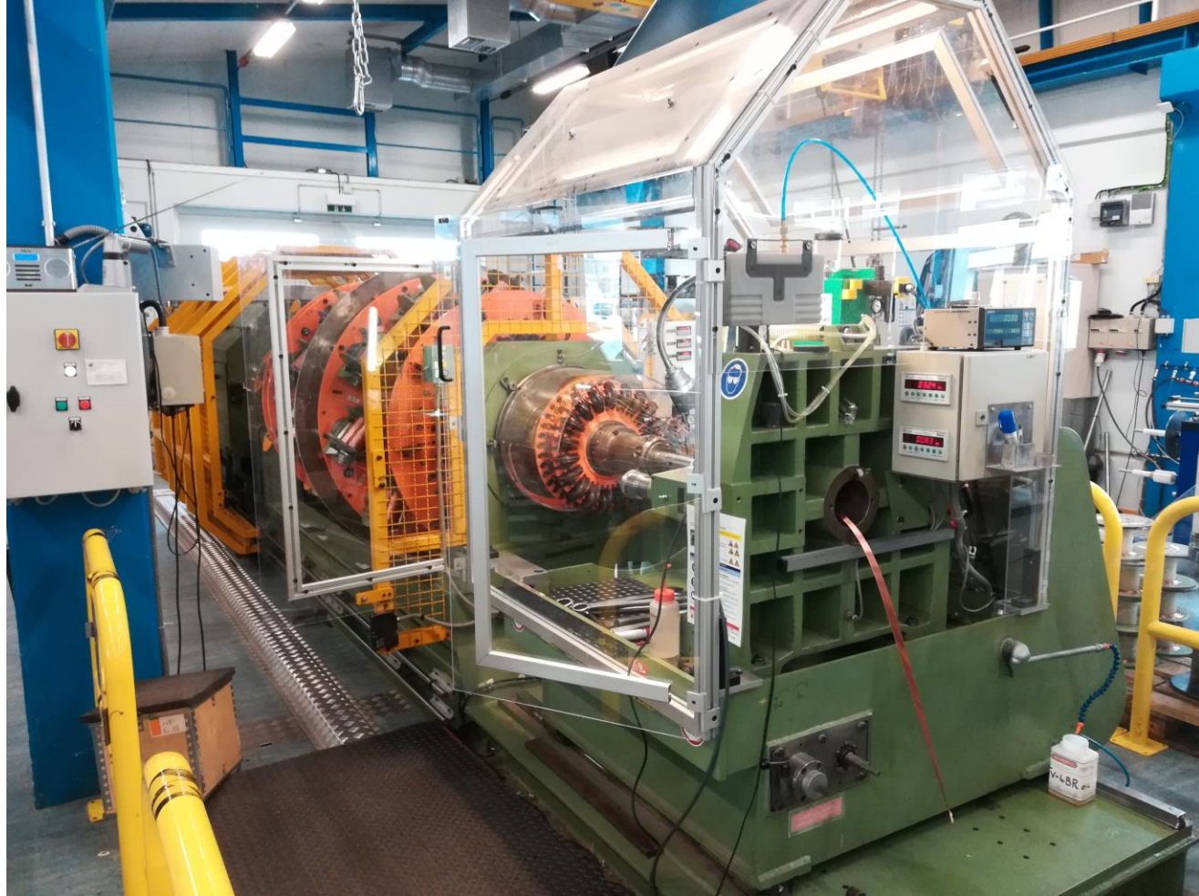
cabling machine (building 163)
