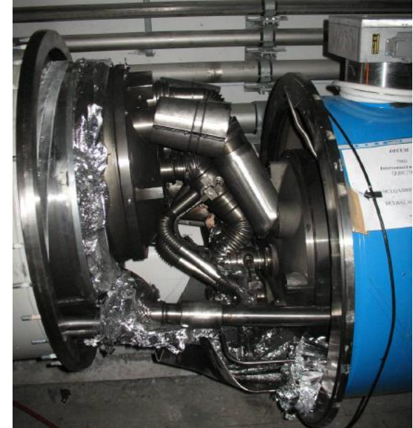
Damage at an LHC interconnect
