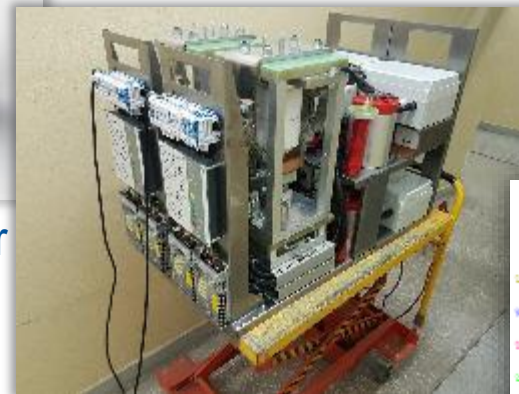
Two vacuum breaker sliding cassettes
