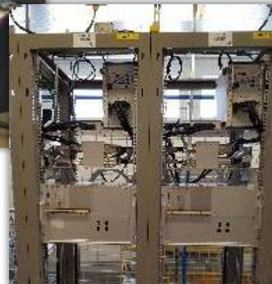
13kA RB and RQD EE systems
