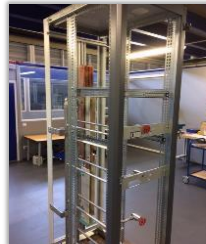
The rack with the busbars and the cooling water pipes
