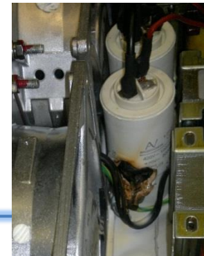
Capacitor starting to burn switched off by DSS
