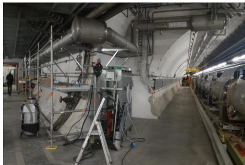
Cryogenic distribution line
