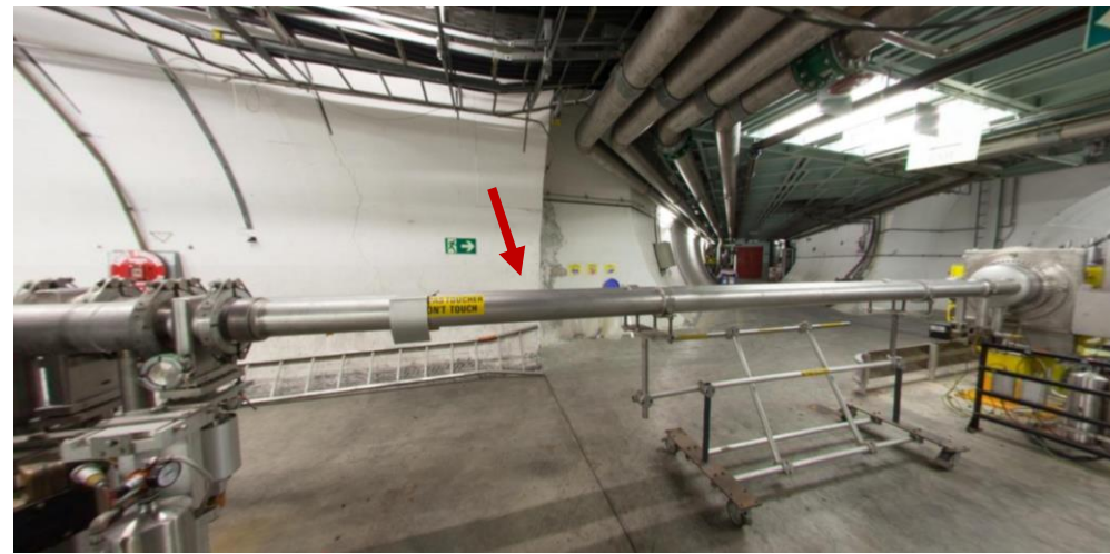
Extraction zone vacuum line
