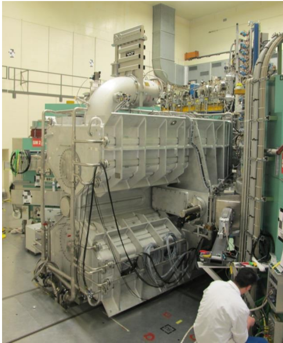
Cabling: All cables from the bunker to outside were installed during shutdown 2018
