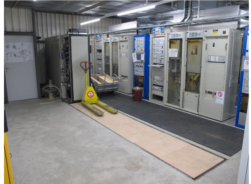
Racks removed. LLRF rack for resonator 4 still in use.
