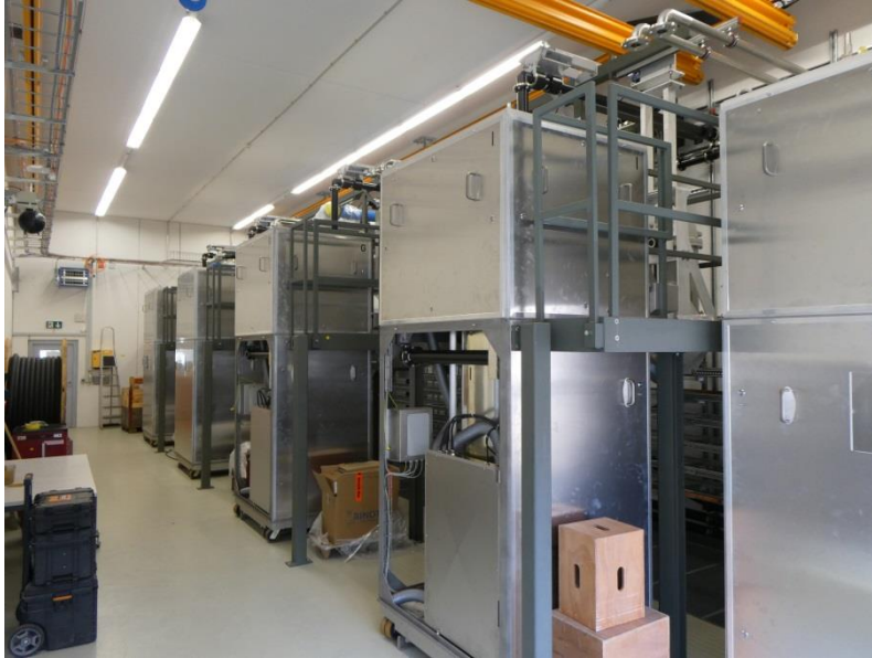
Power amplifiers installed on ground floor WHFA
