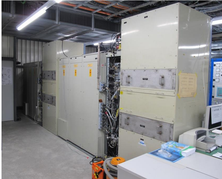
Rack of LLRF for resonator 2 and 1kW / 8kW amplifier chain including air cooling
