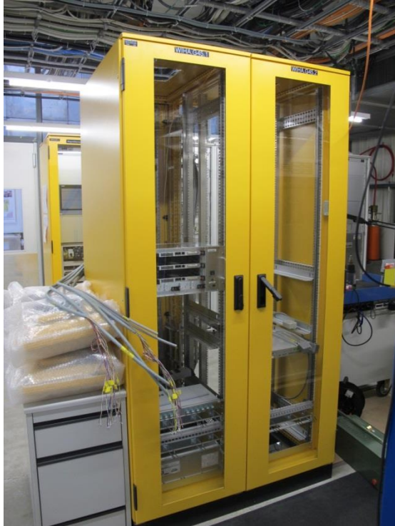
Installation for new LLRF system
