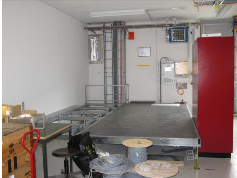
Double floor for 16kV switch gears with interface cabinet, 48V power supply
