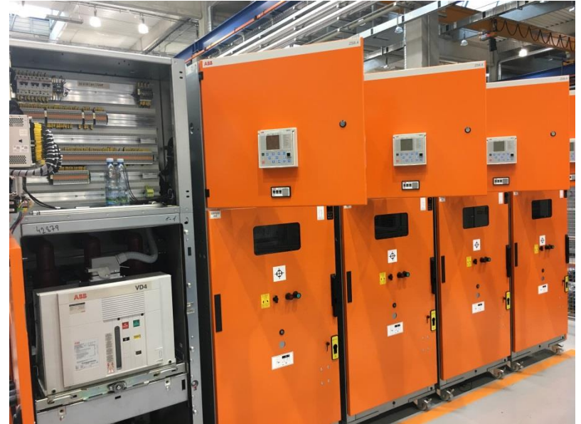
FAT of 16kV switch gears (17./18. May 2018) 5 x ZS8.4 from ABB Delivery and installation at PSI in July
