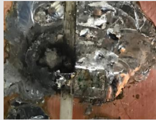
Poor solder of metal cap to cause arc
