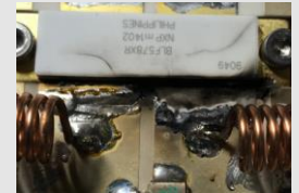
Poor cooling of output PCB and causing the melting of transistor lead
