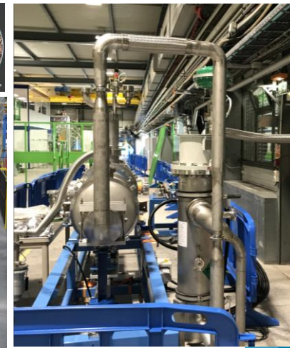
SC links demonstrator test preparation in SM18
