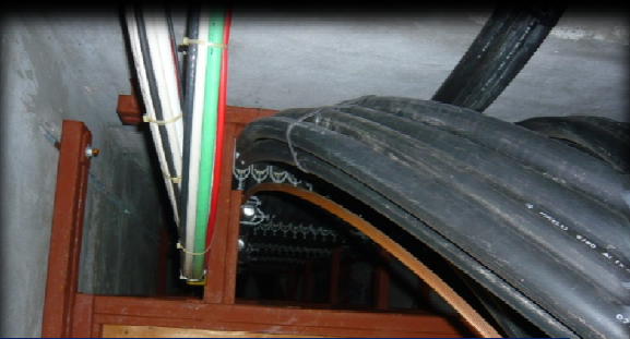
TT7 cable & ventilation shaft
