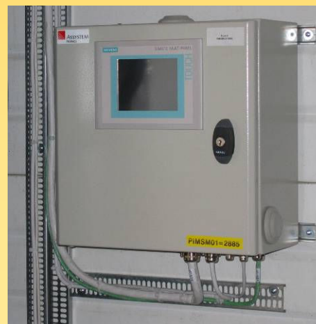
Monitoring station (RAMSES)
