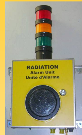
Radiation Alarm Unit (RAMSES)
