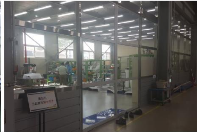
Cleanroom for Storage
