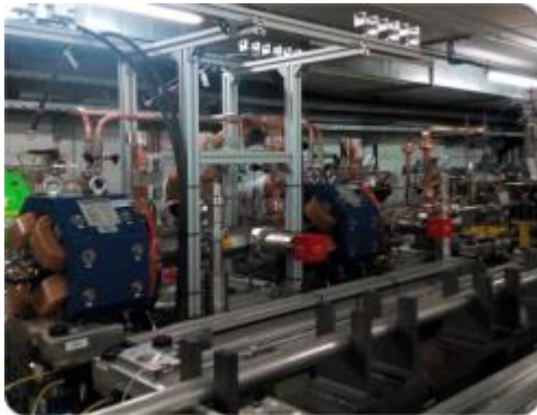
12 Power Extraction Transfer Structures for CTF3
