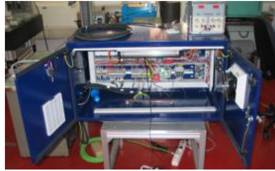
101 Electronic Control Racks
