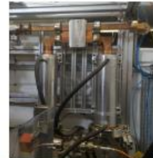
Pulse compressor: provided by CERN
