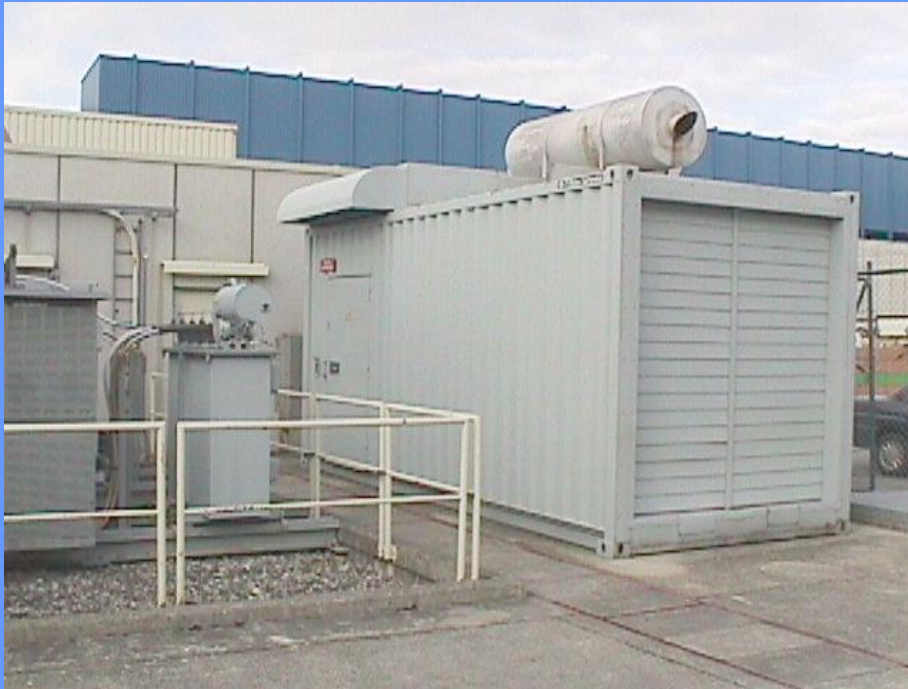
Diesel-generator set 750 kVA, P.A.2
