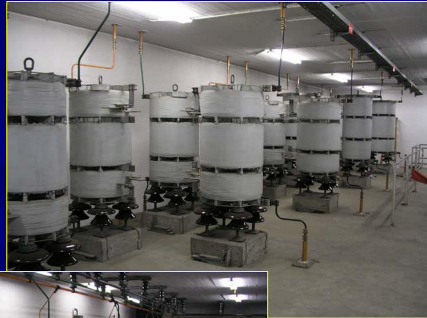
2 nd floor: reactors
