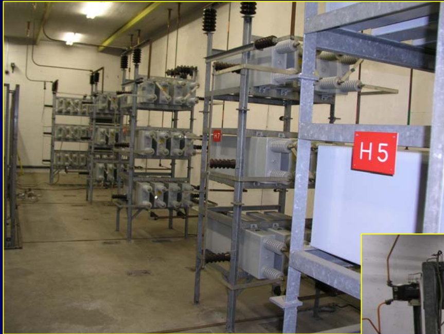
1 st floor: capacitors
