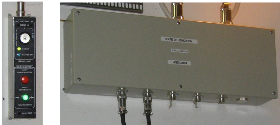
Figure 5 — Sector door opening buttons and patrol box (left) and junction box (right).
