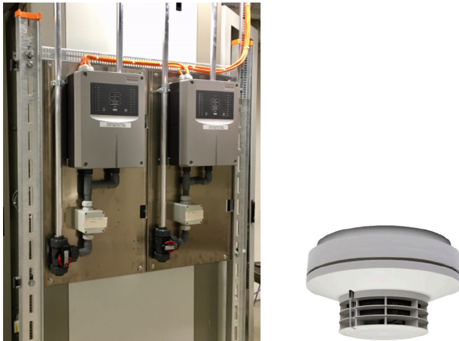
Figure 8 — AFD air sampling smoke detectors (left) and a point detector (right).
