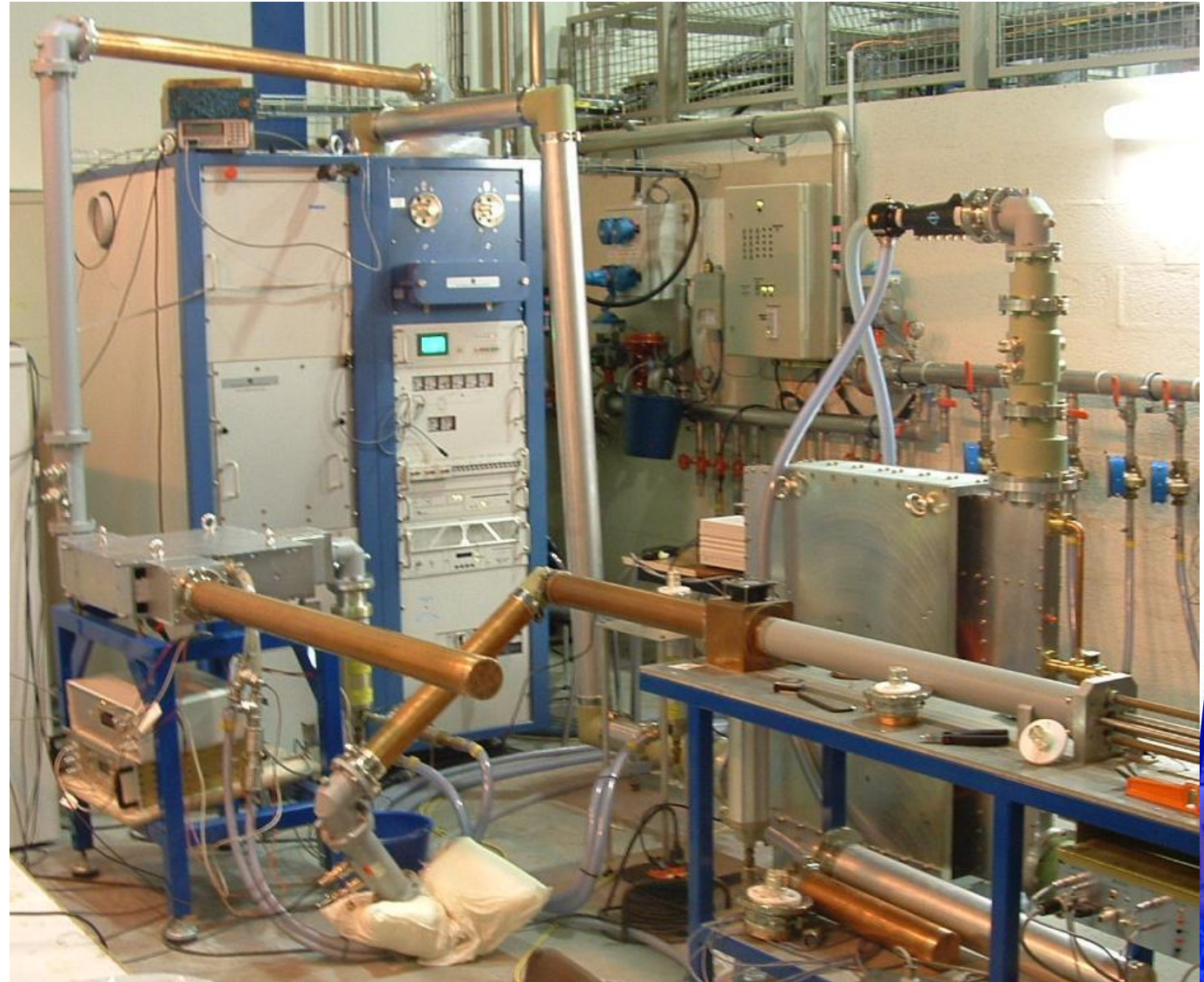
Available parameters: flowmeters, output water temperatures
