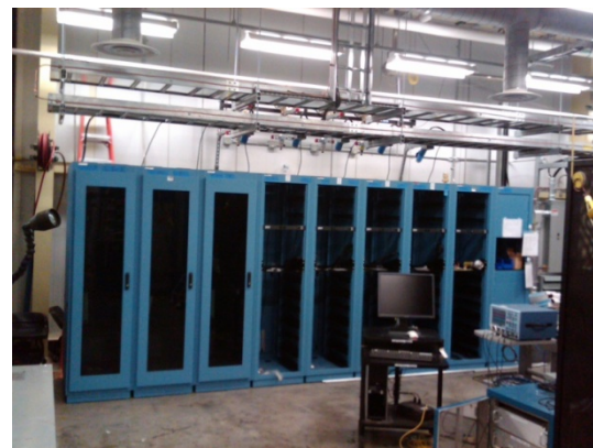
Racks waiting for Amplifiers
