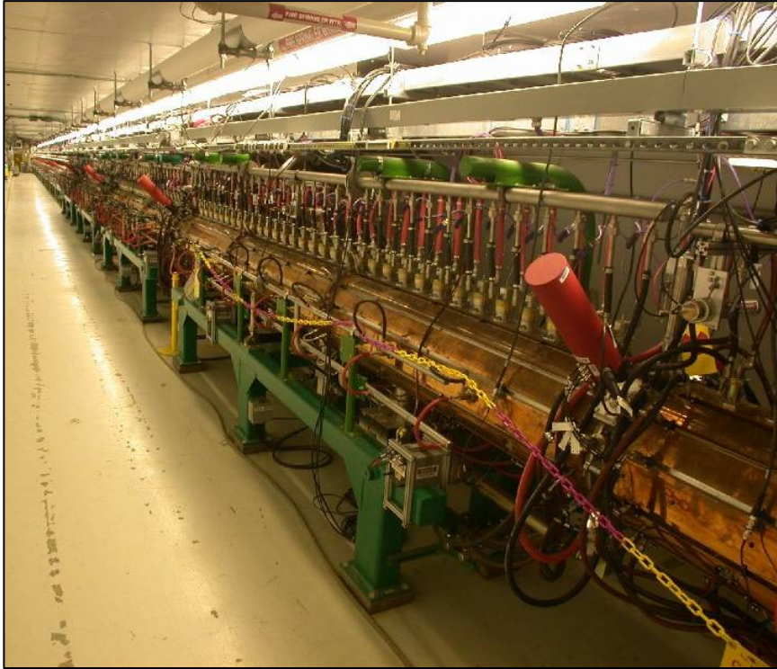
The 402.5 MHz DTL is composed of six sections.
