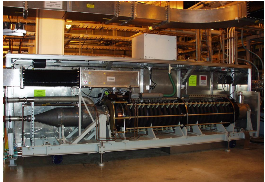
352-MHz/1.1MW CW klystron inside x-ray shield enclosure
