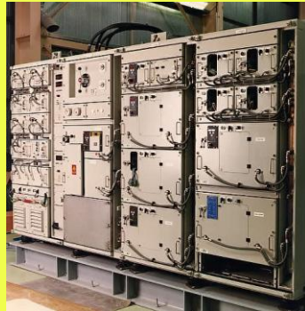
DC-DC Converters Bay
