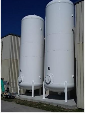
Helium gaz storage
