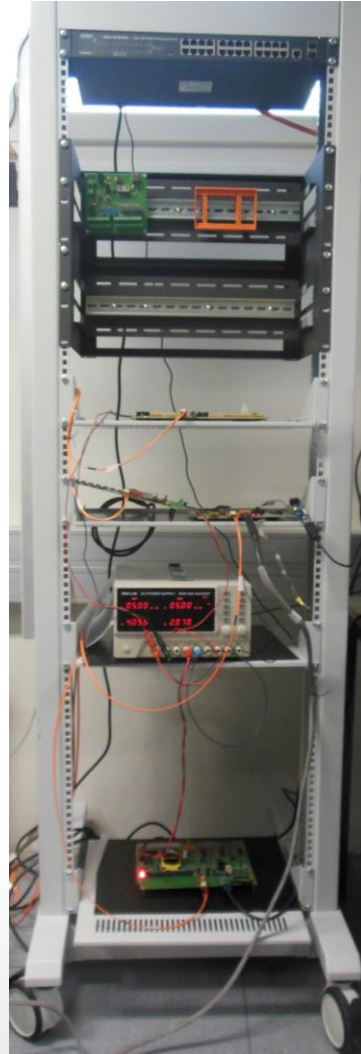
Rack with power supply and boards
