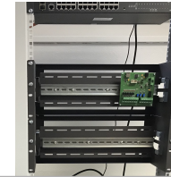
ITS RU in the DCS reference rack
