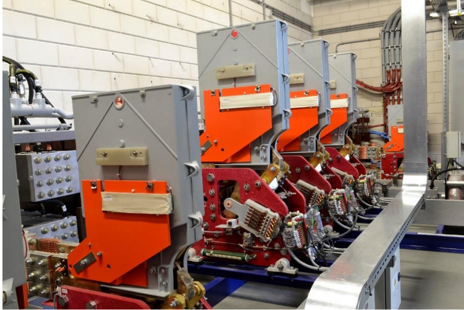
Installation, test and commissioning July 2015
