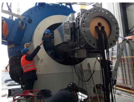
Ecoswing HTS generator
