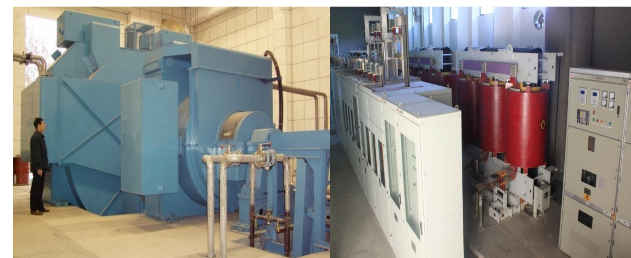
Fig.3. The picture of 100 MVA / 100 MJ Generator and a 67.5 MW rectifier
