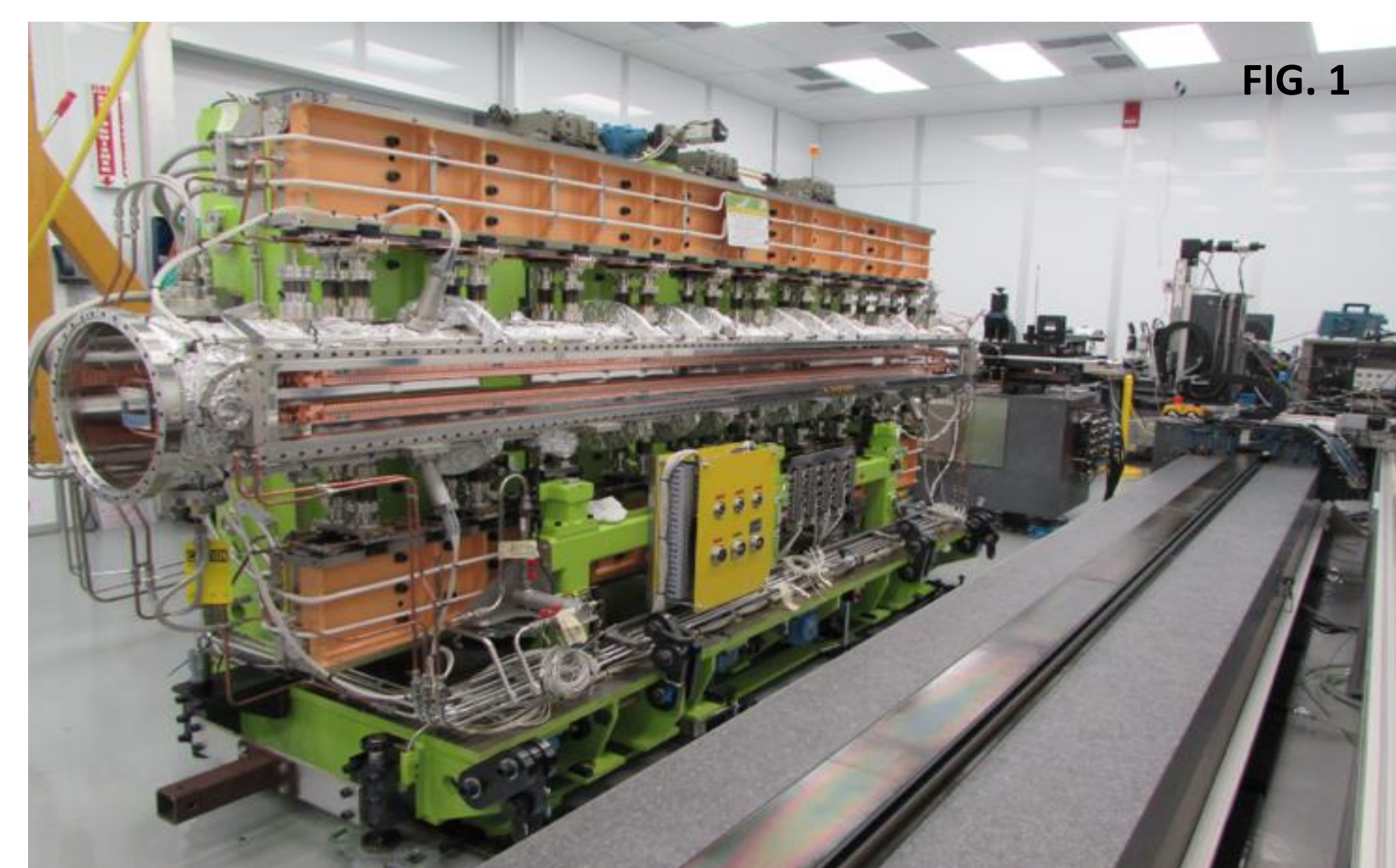
The HXN IVU was procured as turn-key device by Hitachi Metal America (Neomax) and installed into the storage ring in August 2014 in a short straight section. This device has a period length of 20 mm and a maximum effective K of 1.83 at 5.2 mm pole gap. The magnetic module consists of a half period unit with two NdFeB magnet blocks of high intrinsic coercivity and one Permenur pole piece. Figure 1 shows the IVU at the ID magnetic measurement facility (ID-MMF) for magnetic characterization and tuning
