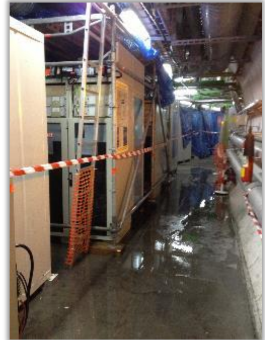
Water leak during LS1
