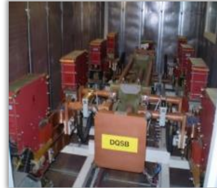
Circuit breakers and busbars
