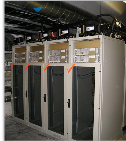
600A EE system racks
