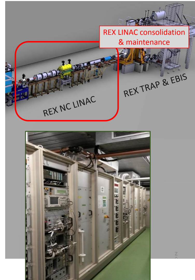
REX RF amplifiers in the REX RF room
