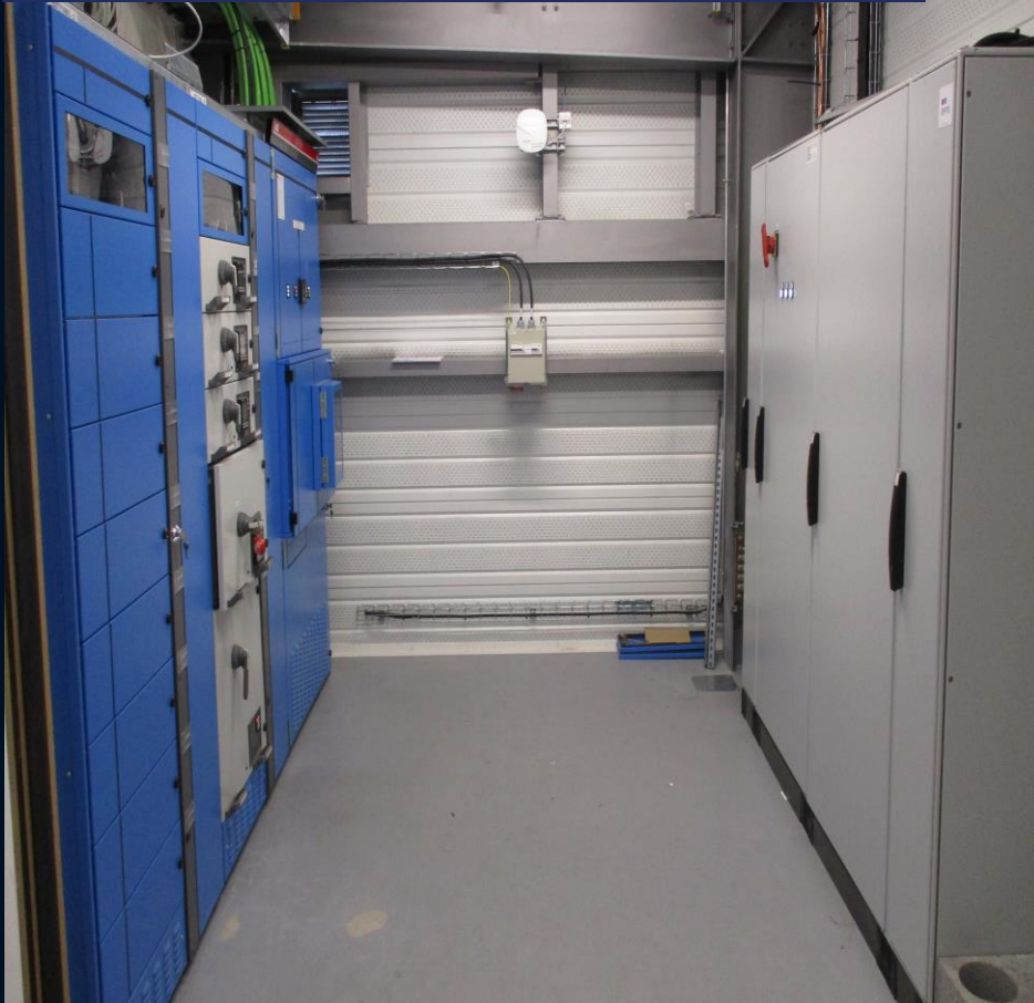
B771 – Electrical installations (2017)
