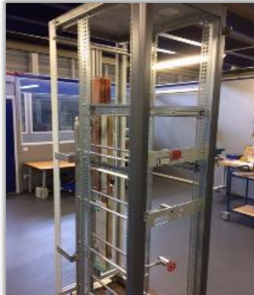
The rack with busbars and cooling water pipes
