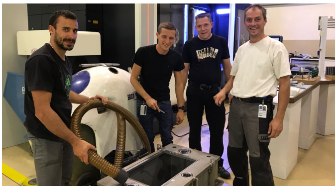
Oil tank for new isolation transformer completed on 26 th September
