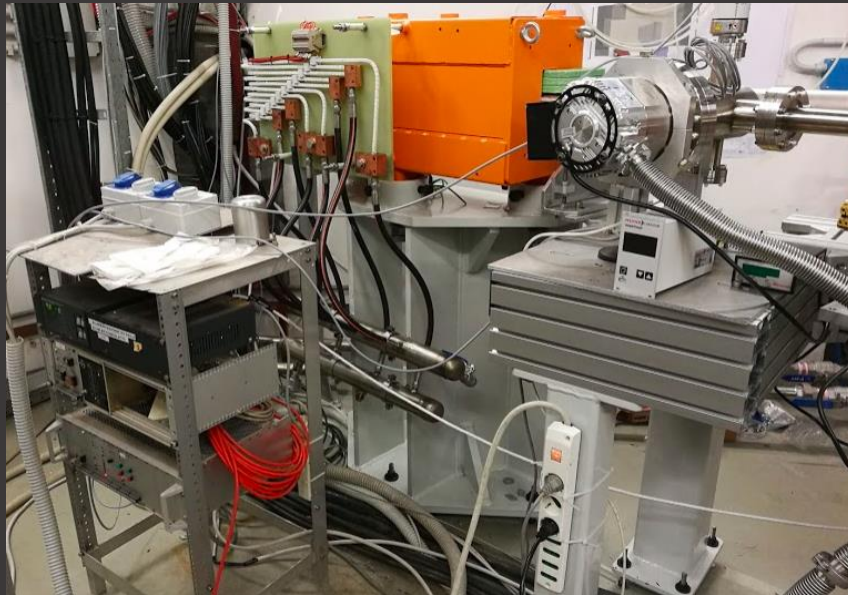
Pumping, gauges, interlock, valves
