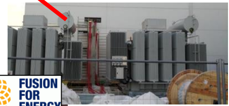
AGPS Conversion system 60MW CW
