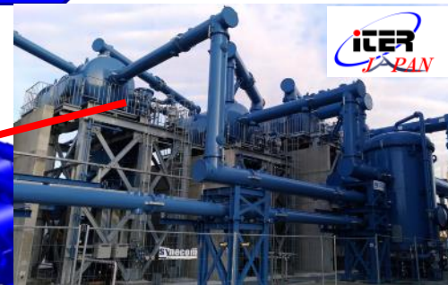
1MV AGPS-DC Generator
