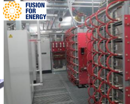
Ion Source Power Supply
