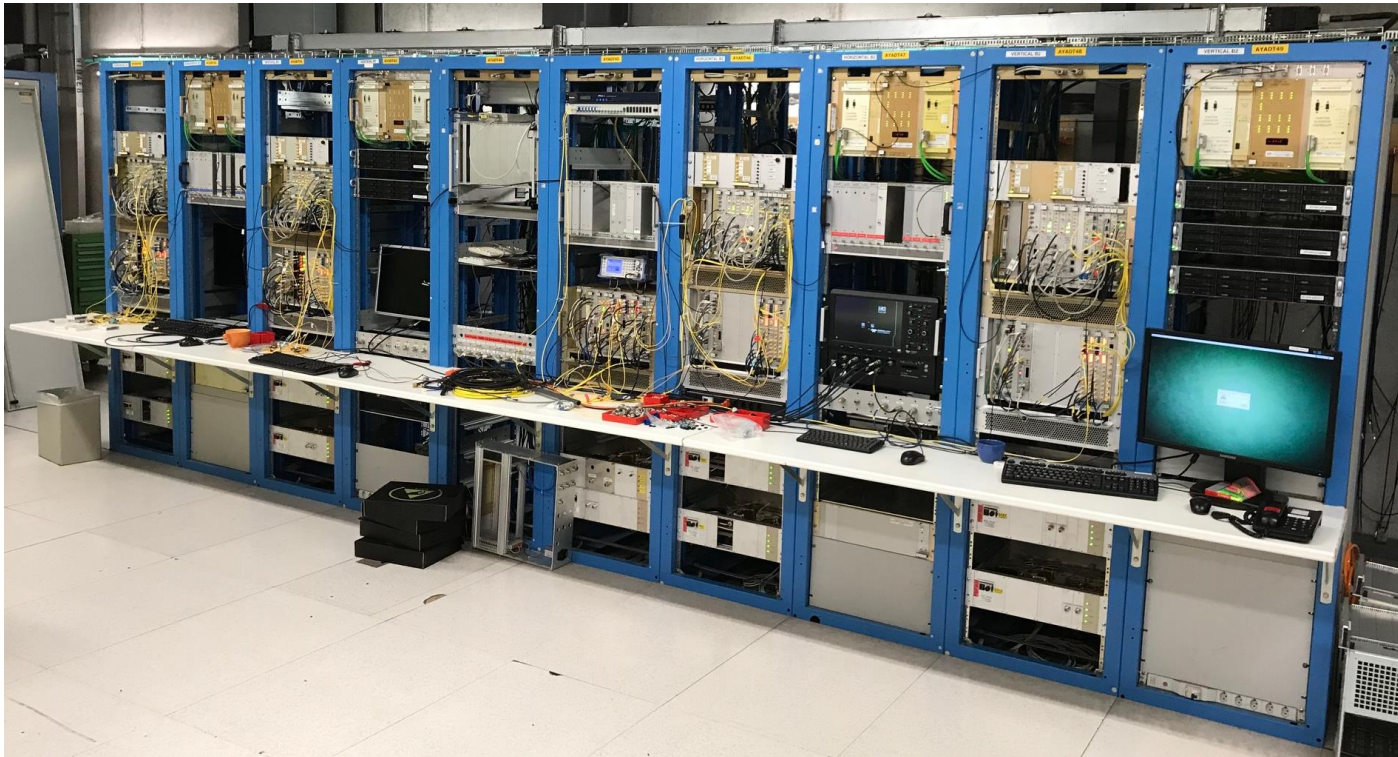
ADT Low Level RF system installed in LHC point 4. Beam position measurement, digital signal processing, all ADTObsBoxes.
