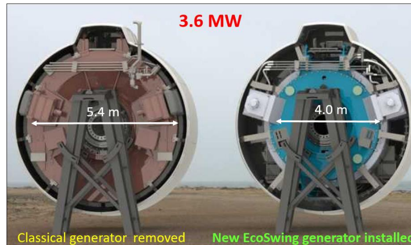
Old and new generator in same casing
