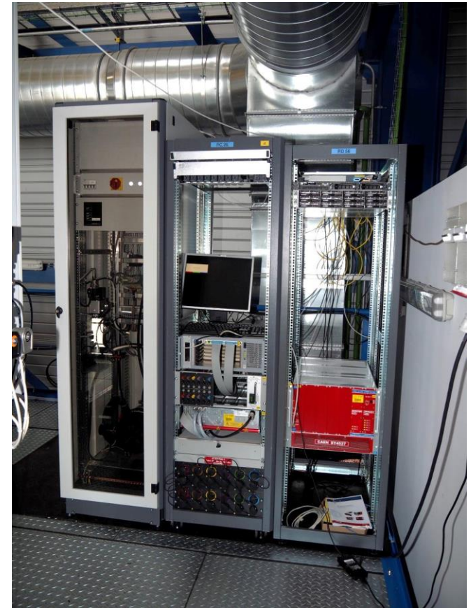
SciFi Vacuum control Rack – Test Frame
