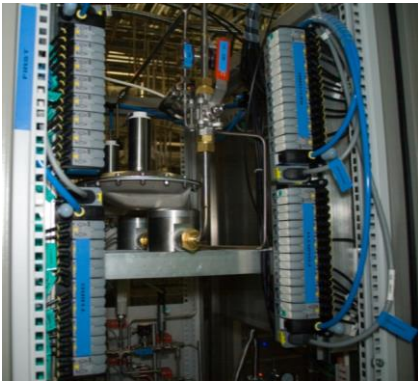
Ar distribution station
