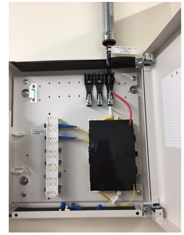
New optical fiber @ server room
