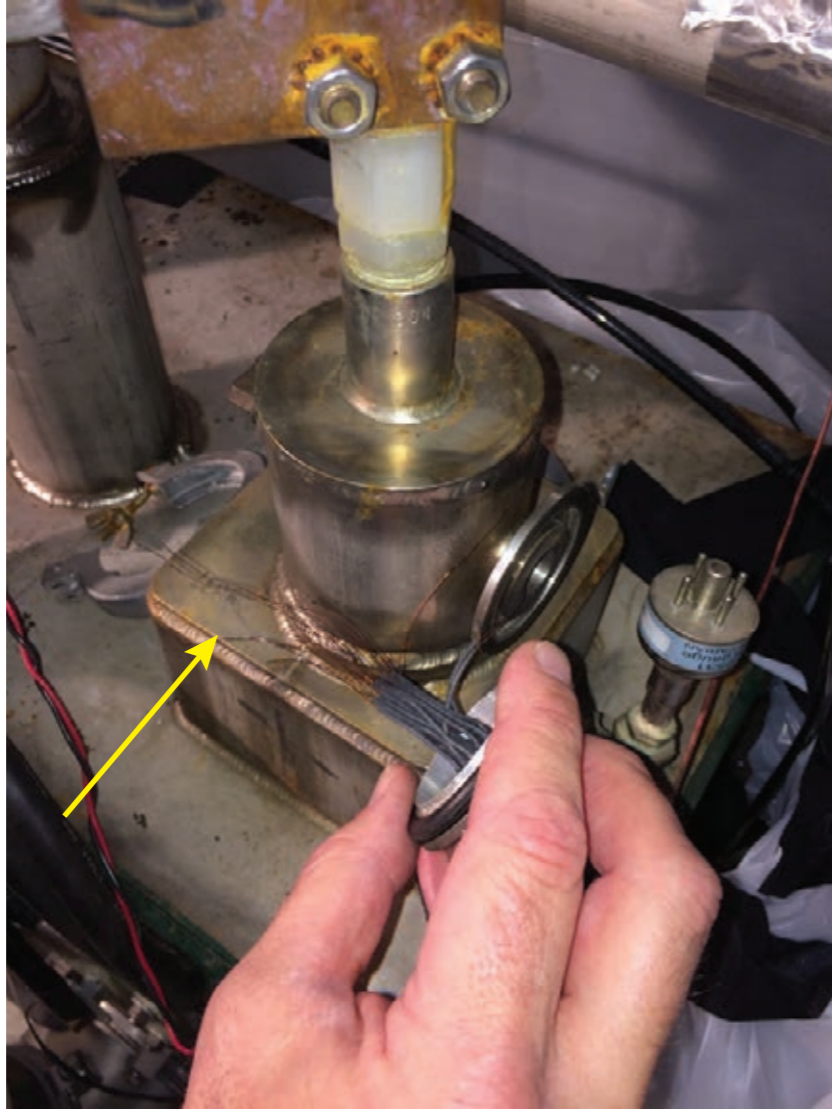
Broken diagnostic wires
