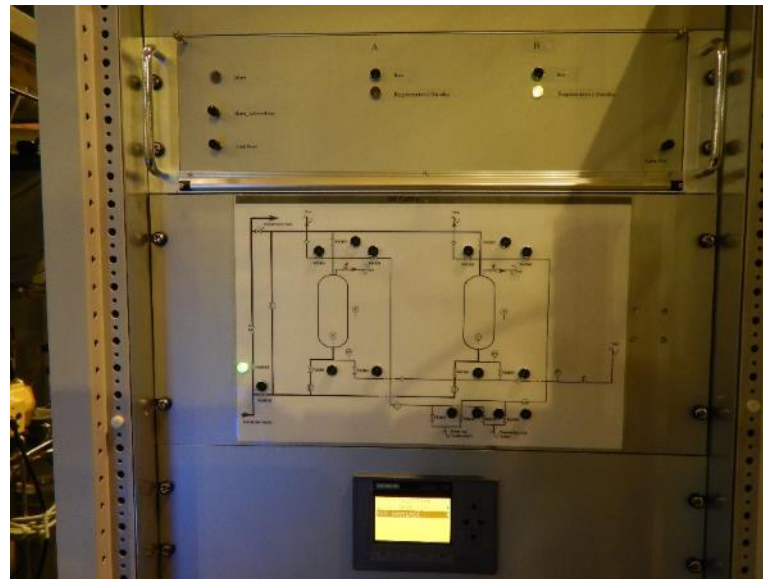
Monitoring and controls panel
