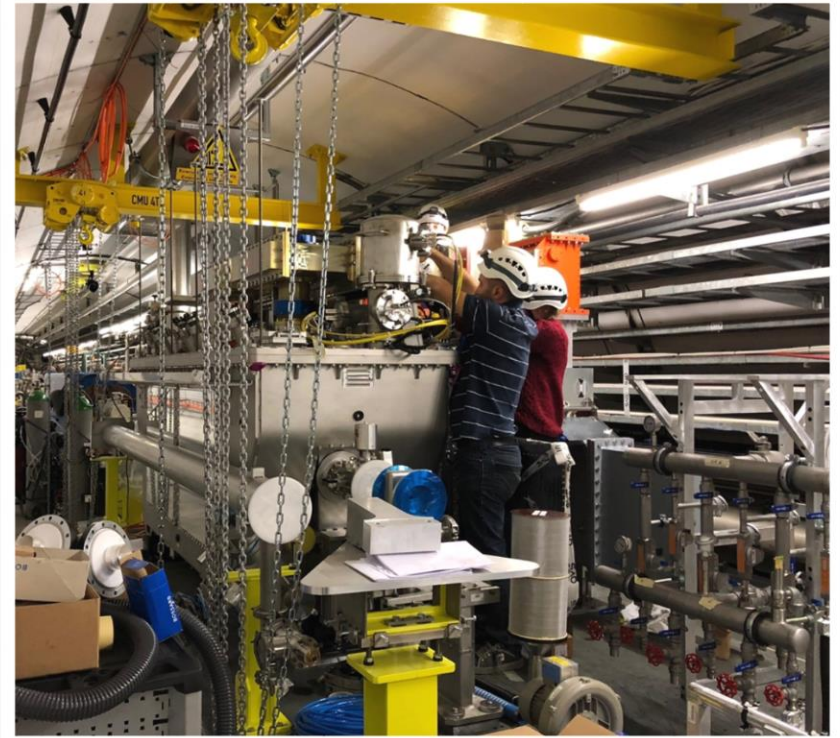
Connection of the FPC to the circulators Antoine, Seb and Frida did very carefully this very sensitive last HPRF action
