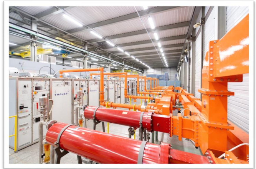
Eight IOT power stations in operation in the SPS since 2014 System availability for beam 99.5 %
